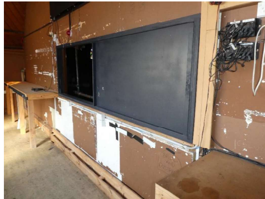
Photograph 146 - Showing the damaged fibrous plaster wall and benching to the meeting / theatre technical room.
