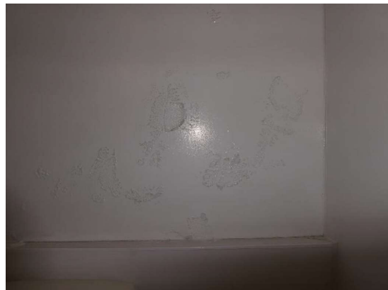
Photograph 129 – Showing the defective paint to the ceiling within the public male toilet.
