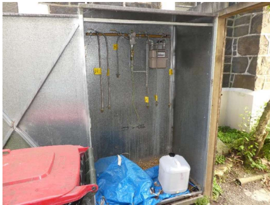
Photograph 261 – Showing the gas bottle storage cupboard to the southern courtyard.
