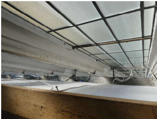
Photograph 168 - Showing the corroded horizontal steel reinforcing and strengthening bars to the inside of the mullioned window.
