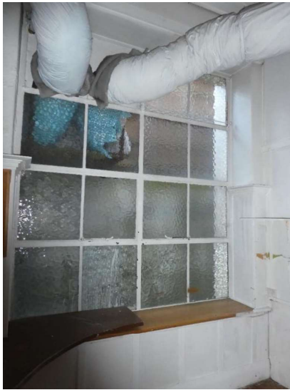
Photograph 255 – Showing poor installation of the insulated warm air ducting to the western basement rooms.
