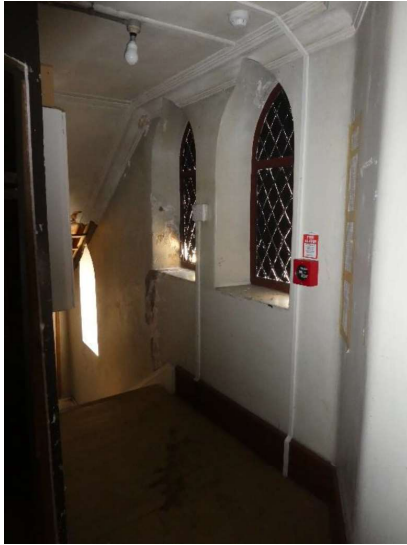
Photograph 176 - Showing the defective plasterwork to the steel ledged lancet windows at the stair landing on the eastern elevation.
