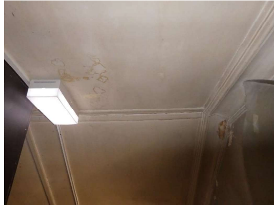
Photograph 115 – Showing typical moisture staining to the original fibrous plaster ceilings.
