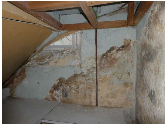
Photograph 164 - Showing the typical condition of the basement walls below the south eastern stairs.
