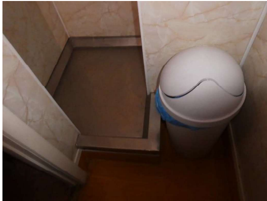
Photograph 224 – Showing the stainless steel shower tray and Seratone linings.
