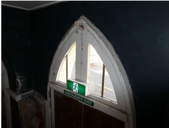
Photograph 192 - Showing the poor condition of the timber lancet top-light window to the south eastern entrance. Noting the maintained fire exit signage.
