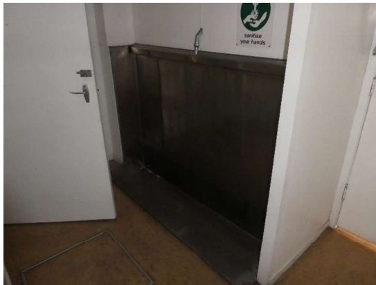
Photograph 229 - Showing the urinal to the male toilet.
