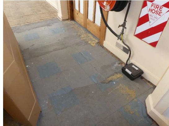
Photograph 132 – Showing the thermoplastic floor tiles to the main entrance foyer. Note these tiles may contain asbestos.
