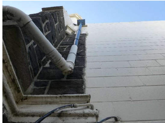
Photograph 18 – Showing the rainwater hopper and iron and uPVC downpipe to the south western corner. Noting the poor detailing between the stone and concrete masonry extension.
