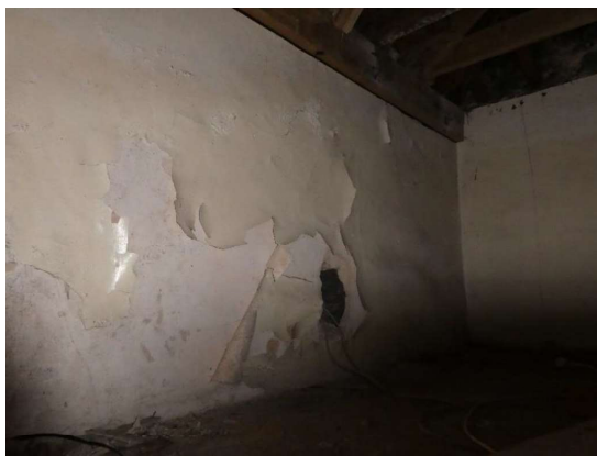
Photograph 65 - Showing the paint failure to the hidden walls within the roof space above the kitchen / bar.
