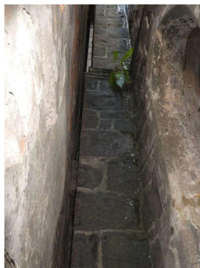
Photograph 34 – Showing the vegetation growth to the western courtyard area.
