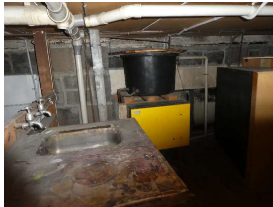
Photograph 263 – Showing the foul water pipework in the south western stairwell. Noting disconnected pipework which requires further investigation.
