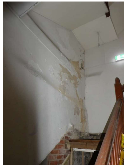
Photograph 206 – Showing the defective plaster within the north western stairwell.
