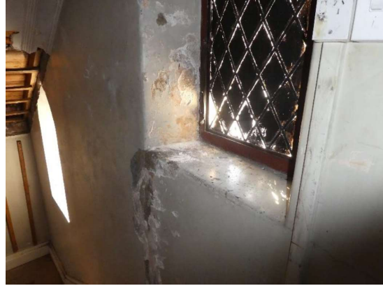
Photograph 177 – Showing the defective plaster and efflorescence to the jamb and sill of the steel ledged lancet windows at the stair landing on the eastern elevation.
