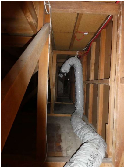
Photograph 259 – Showing the insulated warm air ducting below the seating in the main theatre.
