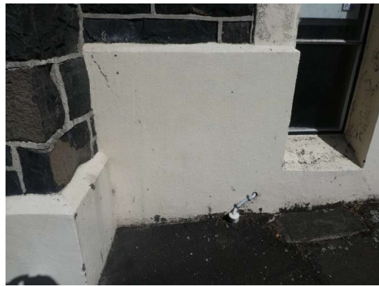
Photograph 245 – Showing the earth stake to the eastern elevation.
