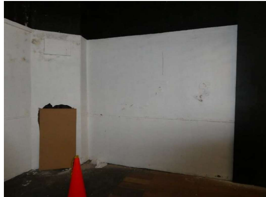
Photograph 151 - Showing the poor condition to the walls and opening within the studio theatre.
