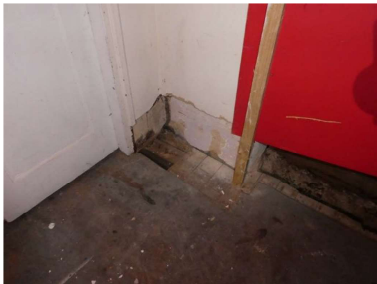
Photograph 205 - Showing defective flooring and low level plaster within the north western stairwell.
