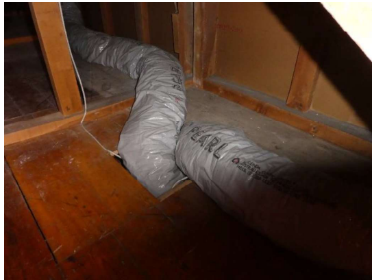
Photograph 257 – Showing the insulated warm air ducting below the seating in the main theatre.
