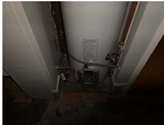
Photograph 251 – Showing the mains pressure gas hot water cylinder housed within the basement toilets.
