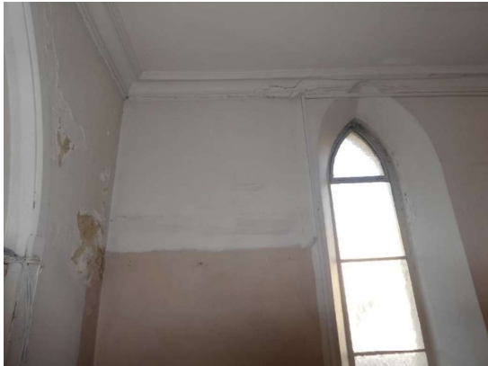
Photograph 150 - Showing the defective plaster to the basement walls within the marketing office.
