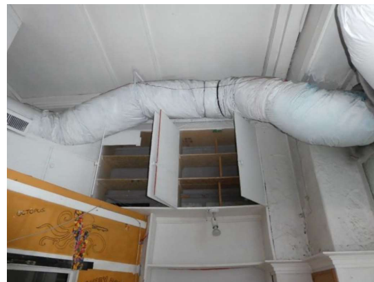
Photograph 254 – Showing insulated warm air heating duct to the western basement rooms.
