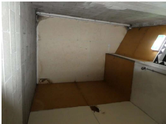
Photograph 128 - Showing the moisture stained ceilings to the south western stairwell.
