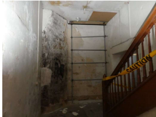
Photograph 202 – Showing the temporary propping within the north western stairwell. Noting unidentified blackspot mould to the plaster walls
