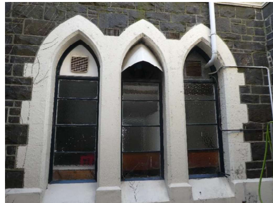
Photograph 51 – Showing the steel framed windows on the western elevation. Noting inappropriate positioning of services.
