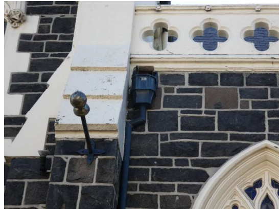
Photograph 16 – Showing the hopper and rainwater downpipe from the south eastern roof.
