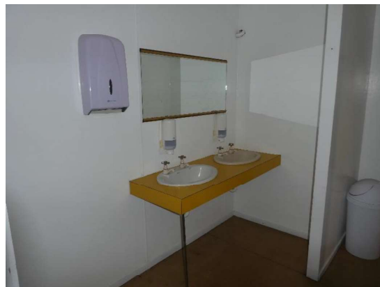
Photograph 232 – Showing the wash hand basins to the female toilet.
