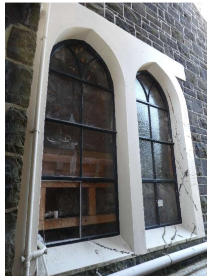
Photograph 63 – Showing the western elevation. Noting corrosion to the steel window frame
