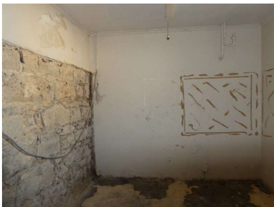
Photograph 152 - Showing the plaster removed from the basement administration office.
