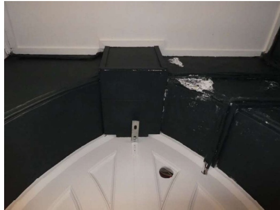
Photograph 193 – Showing the condition of the timber infill panel above the internal doorway to the basement foyer. Noting efflorescence to the solid walls
