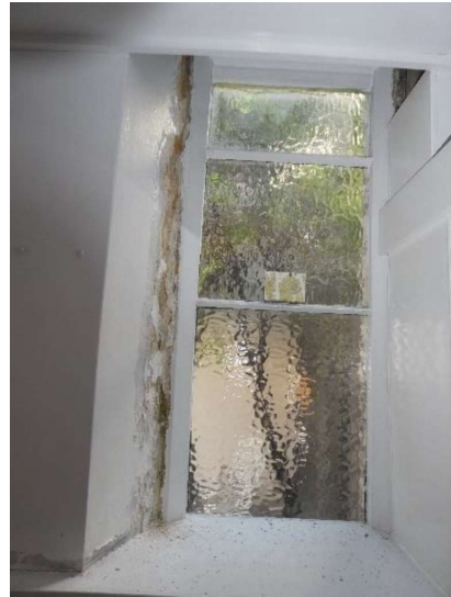
Photograph 185 – Showing the defective paint and plaster to the window in the south western toilets.
