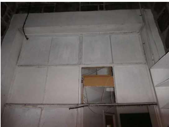
Photograph 186 - Showing the painted windows within the south western stairwell. Noting missing pane.
