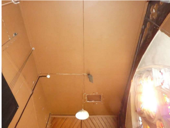
Photograph 114 - Showing the fibrous plaster ceiling to the meeting / theatre technical room. Noting poorly cut and secured roof access hatch.
