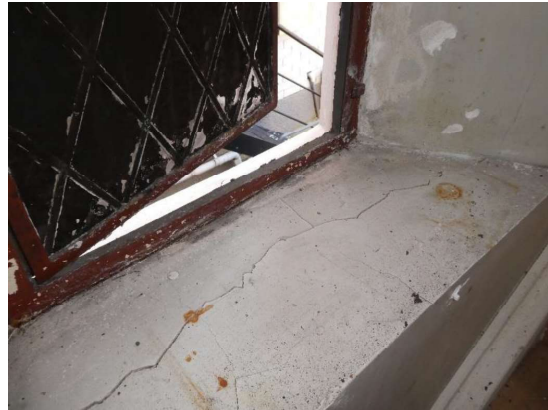
Photograph 179 – Showing the defective cracked plasterwork to the steel ledged lancet windows at the stair landing on the western elevation.
