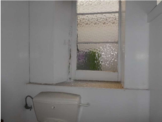
Photograph 184 – Showing the defective paint and plaster to the window in the south western toilets.
