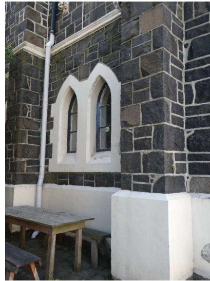
Photograph 53 – Showing the steel framed windows to the south western courtyard area. Noting paint failure, and replacement putty.
