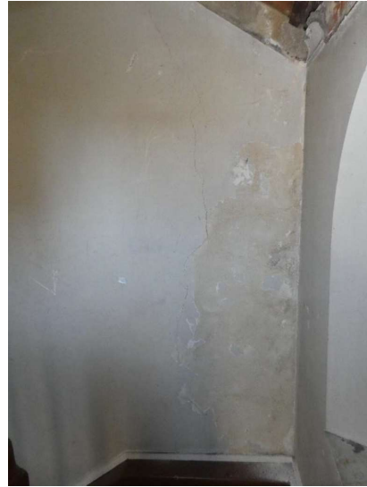
Photograph 149 – Showing the vertical cracking to the plaster wall within the north western staircase.
