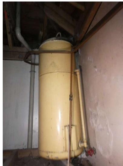
Photograph 249 – Showing the old low pressure hot water cylinder housed within the roof space above the bar / kitchen.
