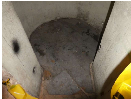
Photograph 156 - Showing the aged vinyl floor covering within the bell tower.
