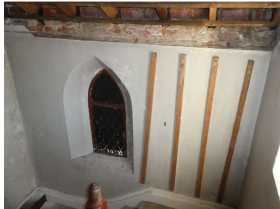
Photograph 117 – Showing typical moisture staining to the original fibrous plaster ceilings.
