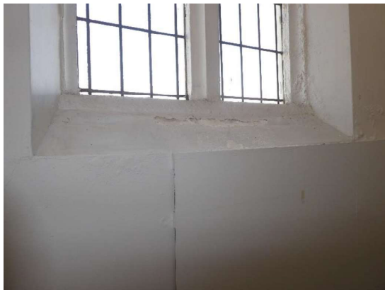
Photograph 180 – Showing the defective paint and plaster to the window sill on the southern wall.
