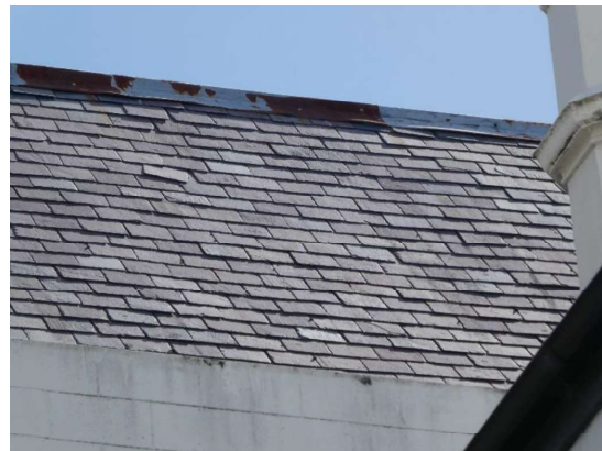
Photograph 4 – Showing the south western roof noting slipped slates and extensive rust to the ridge capping.
